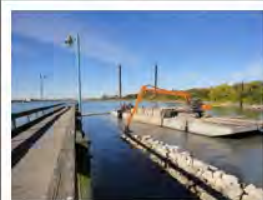
The rocky shoal that blocks wave energy from reaching and eroding the shore of Belle Isle is installed. Photo courtesy of Friends of the Detroit River.
