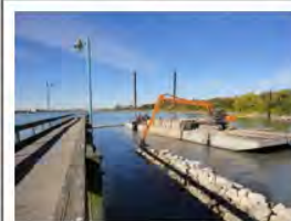
The rocky shoal that blocks wave energy from reaching and eroding the shore of Belle Isle is installed. Photo courtesy of Friends of the Detroit River.
