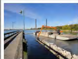
The rocky shoal that blocks wave energy from reaching and eroding the shore of Belle Isle is installed. Photo courtesy of Friends of the Detroit River.
