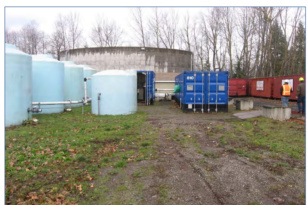
Picture 3. Industrial Facility Discharging to the Columbia River
