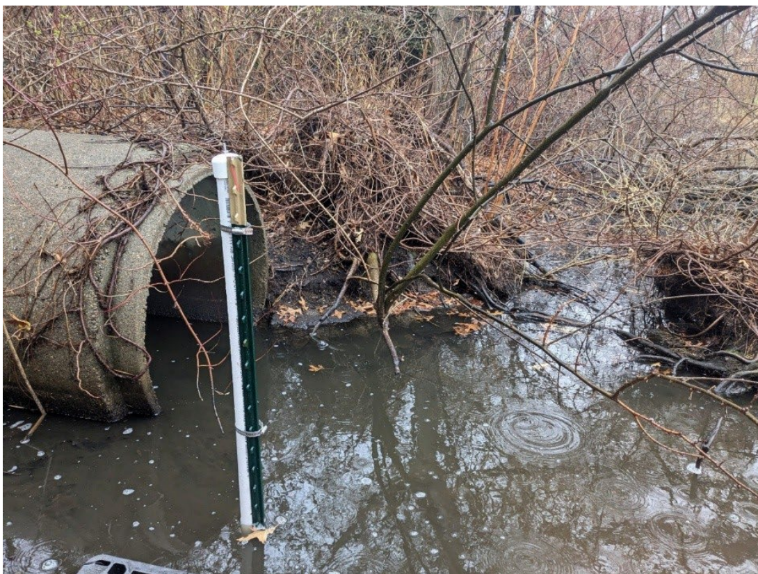
Installation of water level monitoring infrastructure to evaluate hydrologic exchange between the Zoo Wetland and Polo Lake.
