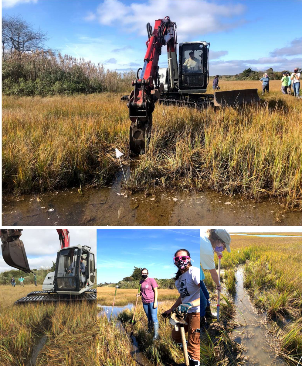
Figure 7. Creation of runnels at Ocean View Farm. Top and Bottom Left: Bristol County Mosquito Control operator creates a runnel with a low-ground pressure excavator. Bottom Center: Staff and volunteers hand-dig a runnel. Bottom Right: Wenley Ferguson hand digs a runnel. Photos: R. Jakuba, A. Besterman, W. Ferguson.
