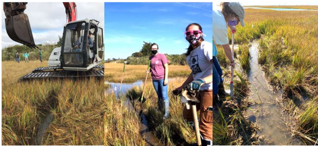
Figure 3. Creation of runnels at Ocean View Farm. Top and Bottom Left: Bristol County Mosquito Control operator creates a runnel with a low-ground pressure excavator. Bottom Center: Staff and volunteers hand-dig a runnel. Bottom Right: Wenley Ferguson hand digs a runnel. Photos: R. Jakuba, A. Besterman, W. Ferguson.
