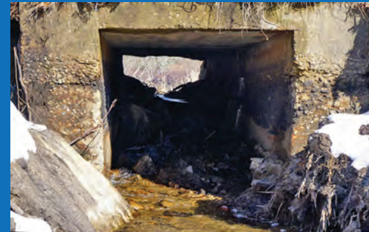
Early February 2021 – Deteriorated Culvert
