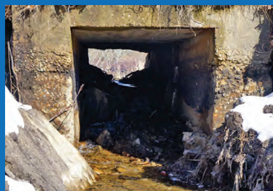
February 2021 – Deteriorated, Blocked Culvert
