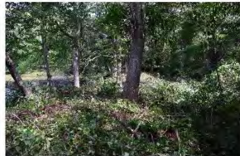
At right, view of the top of the earthen (primary) dam, looking east.
