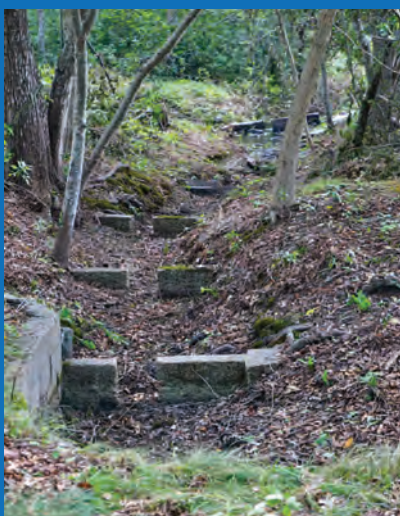
August 2020 Non-functional Fish Ladder
