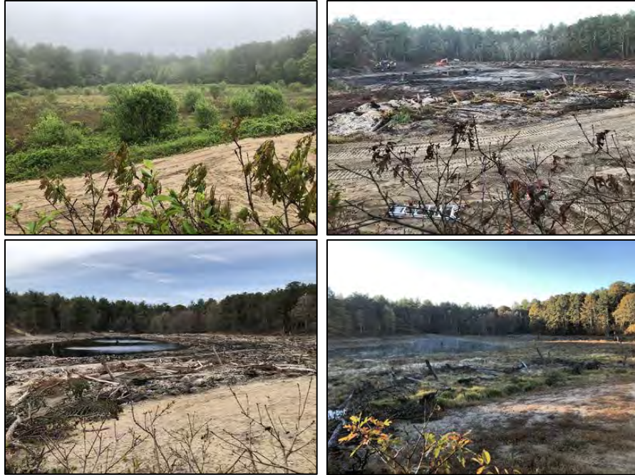
Eastern Garner Bog picture post images May and November 2020 (top left and right) and 2021 (bottom left and right) showing progression of work from before, during and after construction. Photo credit: FRGC.
