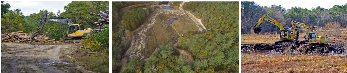
Construction in the bogs including installation of woody material and creation of the new stream channel and ponds for waterfowl. Photo Credits: FRGC and Inter-Fluve.
