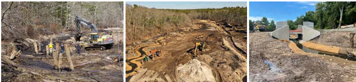
Construction of the new river channel through the former impoundments and installation of the new culvert at Carriage Shop Road. Photo credits: Inter-Fluve.
