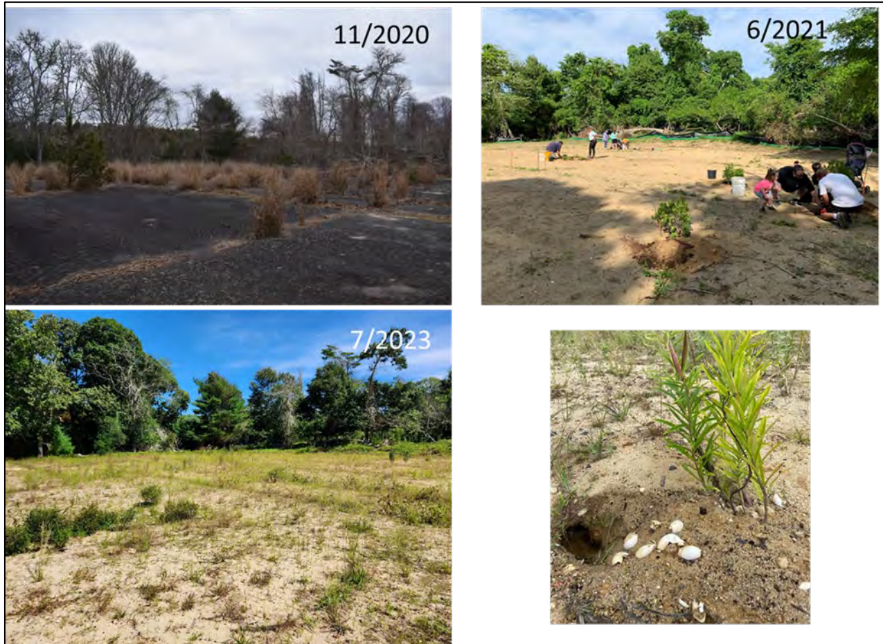
Figure 5. Reference photos of the conversion of an asphalt shuffleboard court to turtle nesting habitat at Great Neck. The asphalt was removed in the winter 2021 and the photos in the left column show the area pre- and post-restoration. Over 90 native shrub and flower transplants were planted by volunteers in the summer of 2021, shown in the upper right photo, and nesting turtles were detected one year after restoration. Hatched turtle eggs and nest are shown in the lower right photo.
