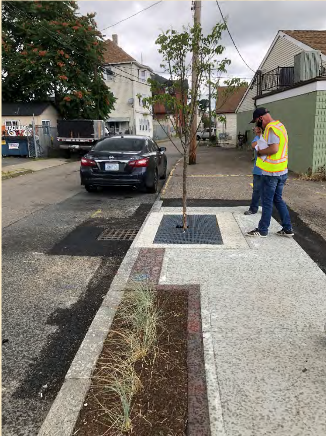
New Tree Filter w/ attached catch basin & new sidewalk planting bed on Chaffee
