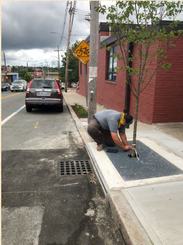
New Tree Filter w/ attached catch basin
