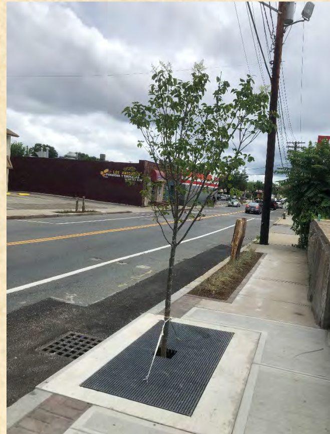
New Tree Filter w/ attached catch basin (close-up)
