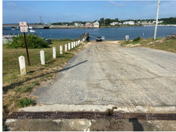
Figure 8: Electric Avenue Boat Ramp and Buttermilk Bay. Note failed stormwater drain in foreground. Photo credit: APCC.
