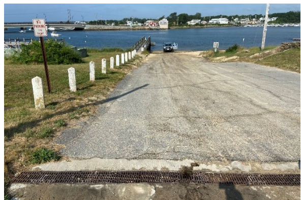
Figure 7: Electric Avenue Boat Ramp and Buttermilk Bay. Note failed stormwater drain in foreground. Photo credit: APCC.
