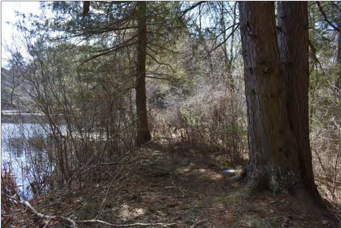
Photo 6. Overgrown earthen crest of the Capwell Mill Pond Dam, view south.
