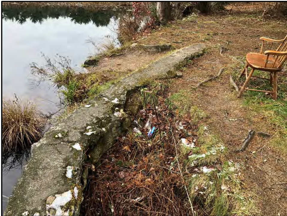
Photograph 2-4. Horizontal cracking across top of concrete portion of left embankment wall at the impoundment and large scour hole in bottom center of photograph. Looking southeast.
