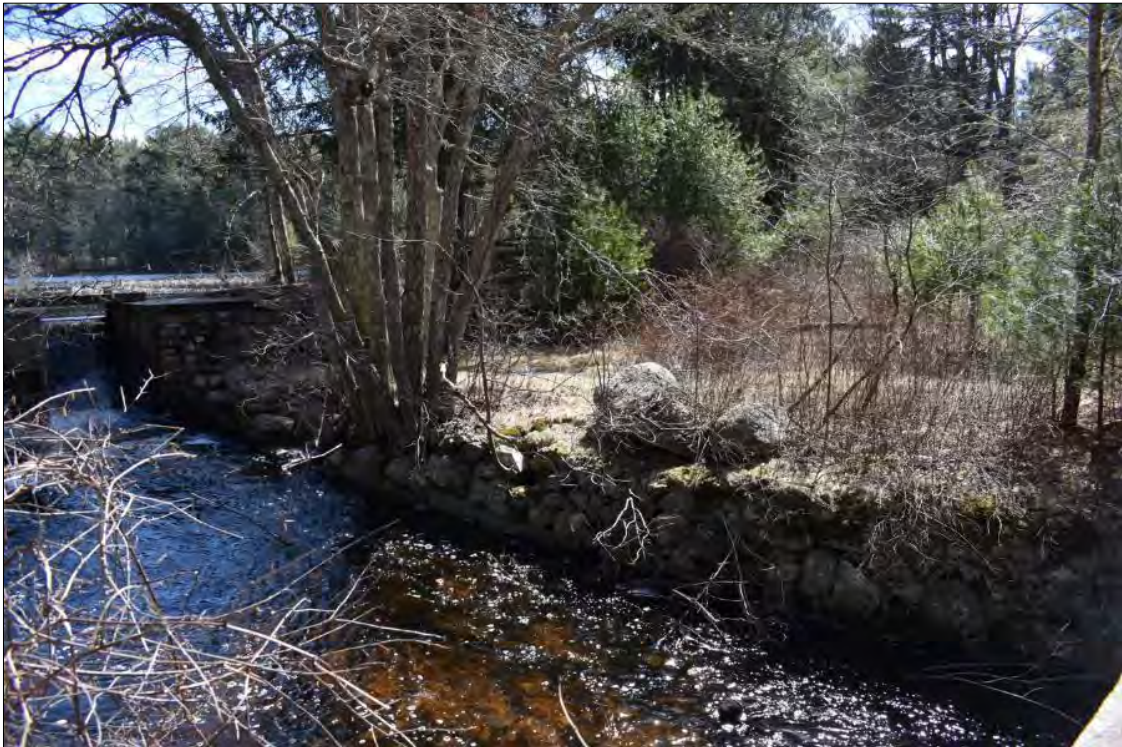
Photo 15. Stone-lined river wall on the south bank of the Carr River downstream from the Capwell Mill Pond Dam, view southeast.
