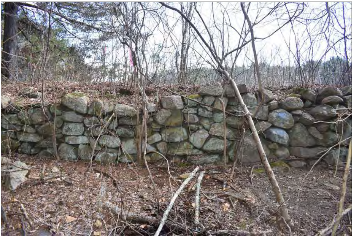
Photo 4. Dry-laid stone masonry on the downstream face of the Capwell Mill Pond Dam, view east.
