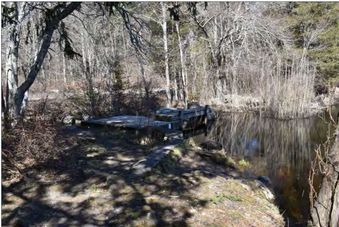
Photo 12. Capwell Mill Pond Dam spillway and sluice with a water level meter on the upstream (east) face, view southwest.
