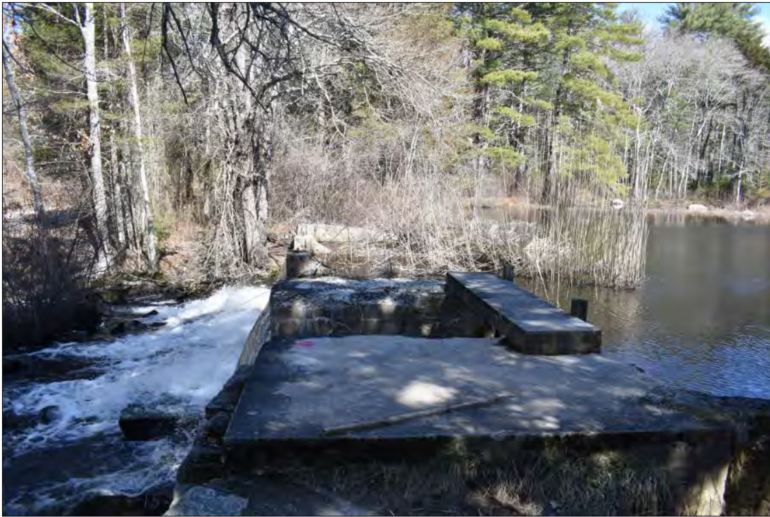
Photo 11. Capwell Mill Pond Dam spillway and sluice with a small wooden footbridge.
