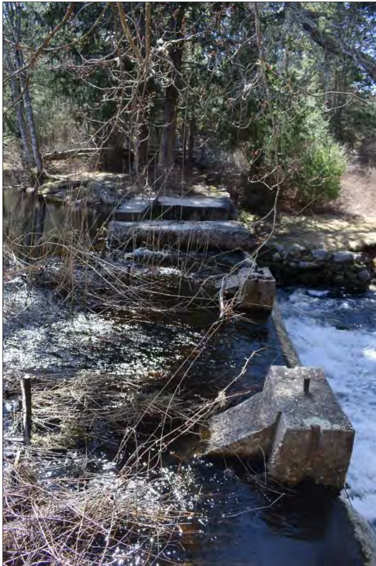
Photo 13. Slatted concrete piers at the spillway of the Capwell Mill Pond Dam, view south.
