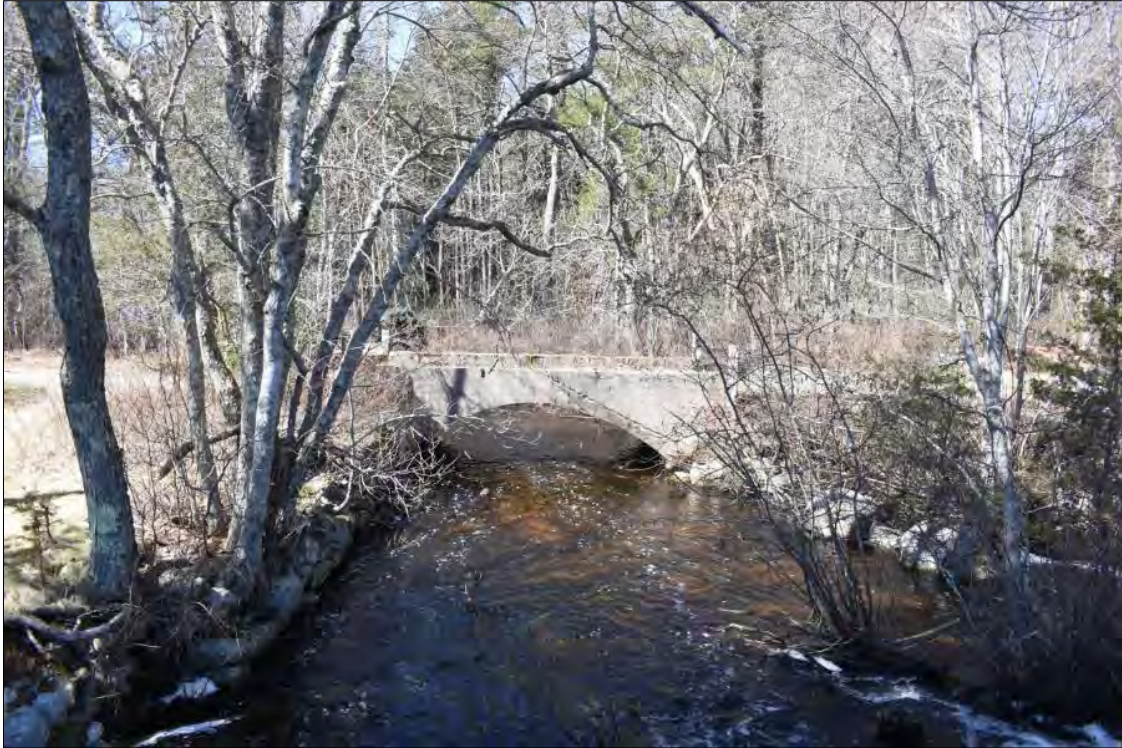
Photo 14. Concrete arch bridge immediately downstream of the Capwell Mill Pond Dam on Burnt Sawmill Road, view west.
