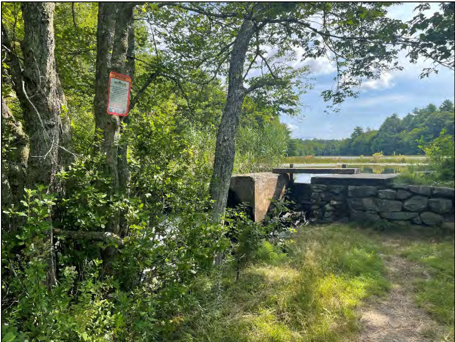
Photo 2: Location of the informational sign relative to the Capwell Mill Pond Dam, looking east
