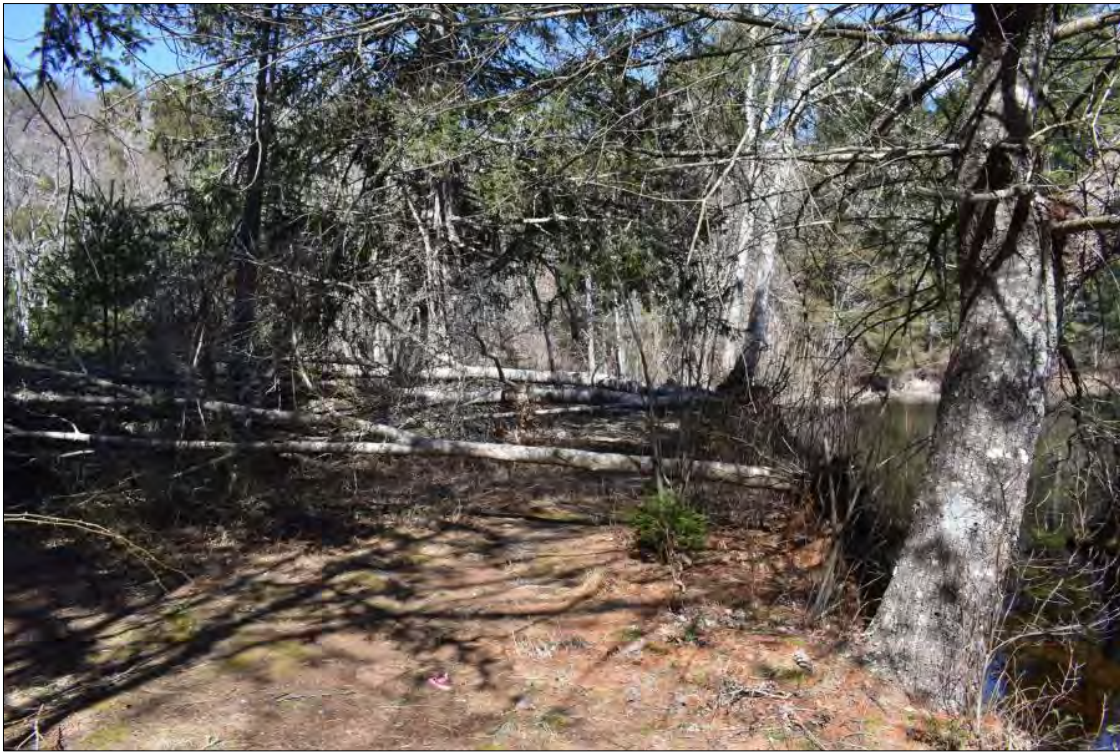
Photo 7. Overgrown earthen crest of the Capwell Mill Pond Dam, view north.
