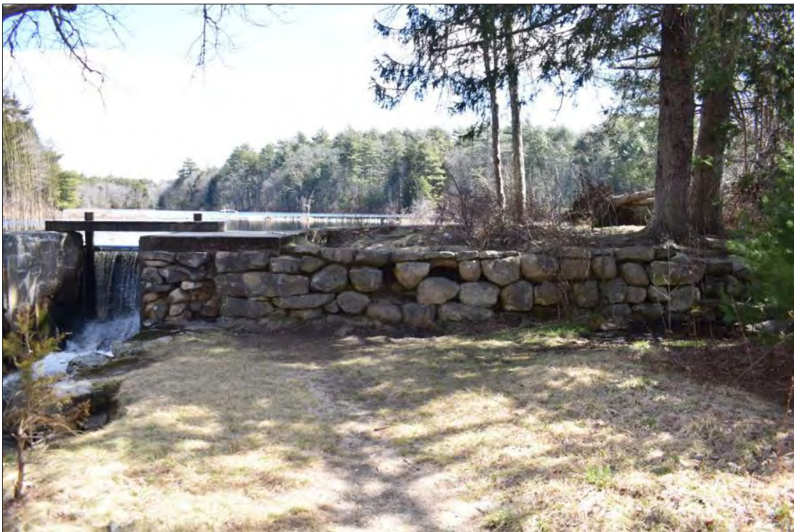
Photo 8. Dry-laid stone masonry on the downstream face of the Capwell Mill Pond Dam, view east.
