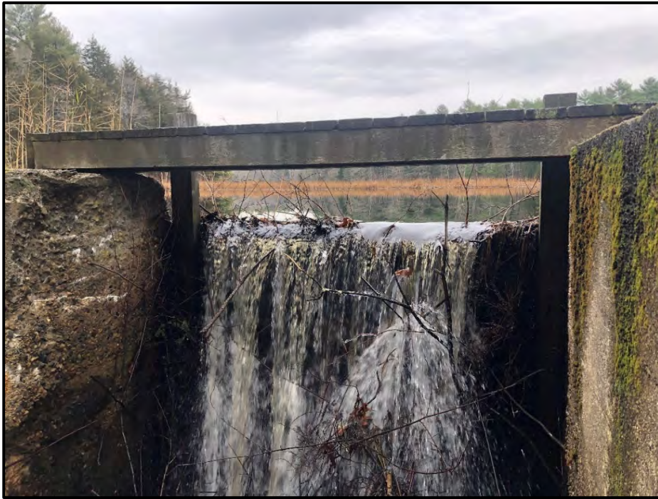
Photograph 2-3. Downstream side of timber low-level outlet at spillway. Flow overtopping timber planks which are secured to vertical timber posts. Pedestrian bridge, spalling of concrete, and accumulation of beaver debris within outlet are shown. Looking east.
