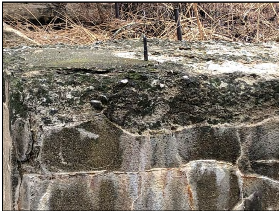
Photograph 2-2. Spalling at top of left concrete sidewall and exposed rebar protruding from concrete. Looking north.
