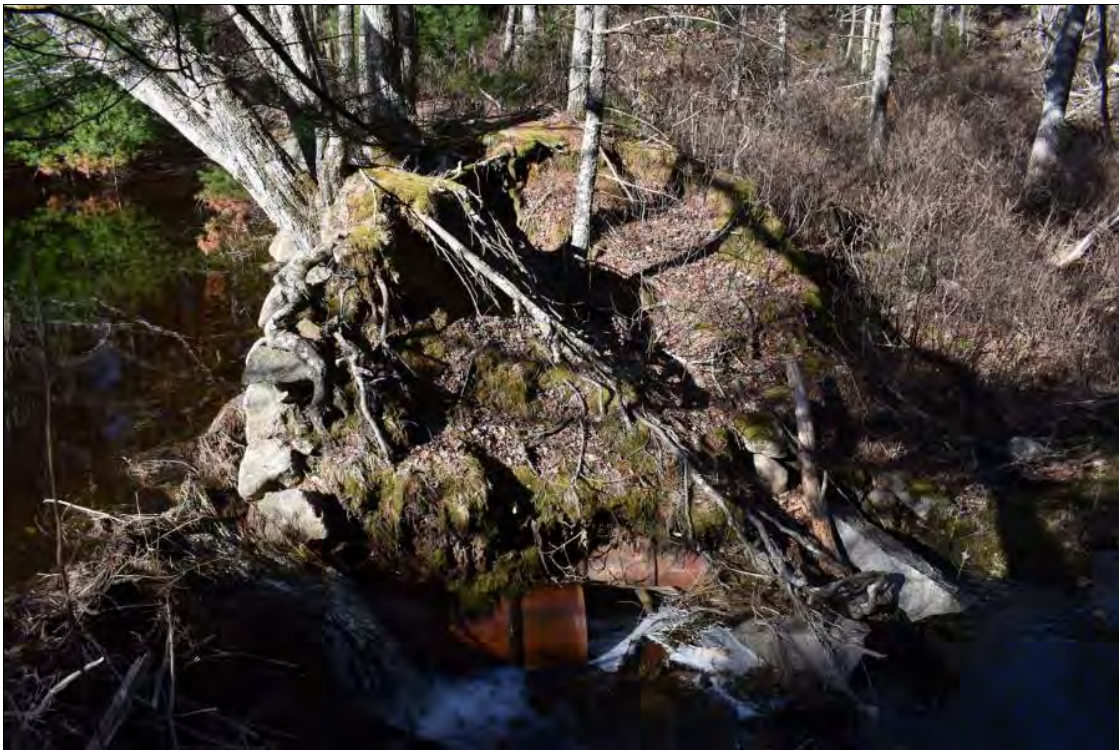
Photo 32. Sweet Pond Dam spillway with ceramic drain pipes and collapsed masonry, view west.
