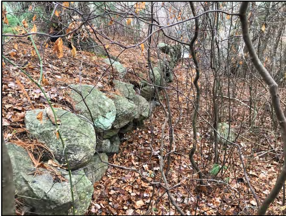
Photograph 2-6. Outward bulge of downstream side of right embankment wall. Large tree in top left corner of photograph. Looking south.
