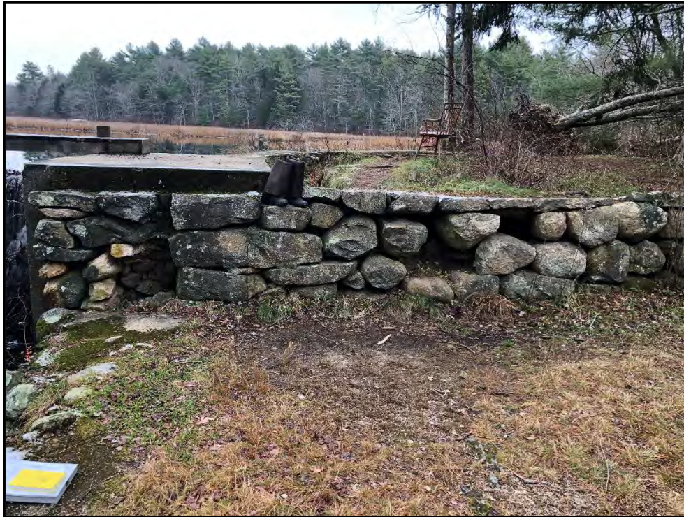
Photograph 2-5. Missing stones/gaps in downstream side of masonry left embankment wall near spillway. Looking east.
