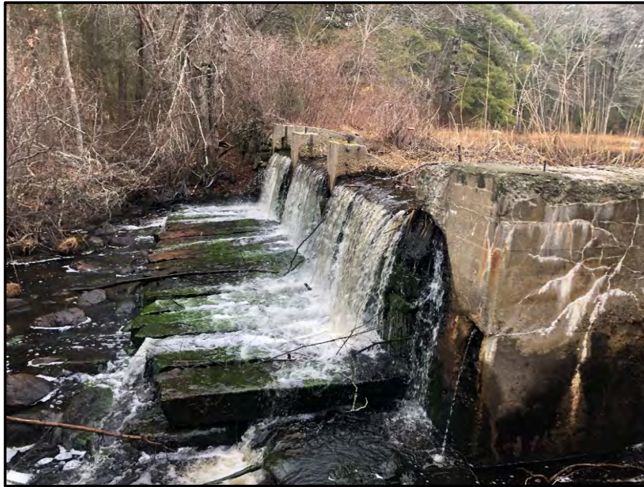
Photograph 2-1. Capwell Mill Pond Dam concrete and masonry spillway. Deterioration of concrete structures and vegetation on right bank of dam evident. Looking north.
