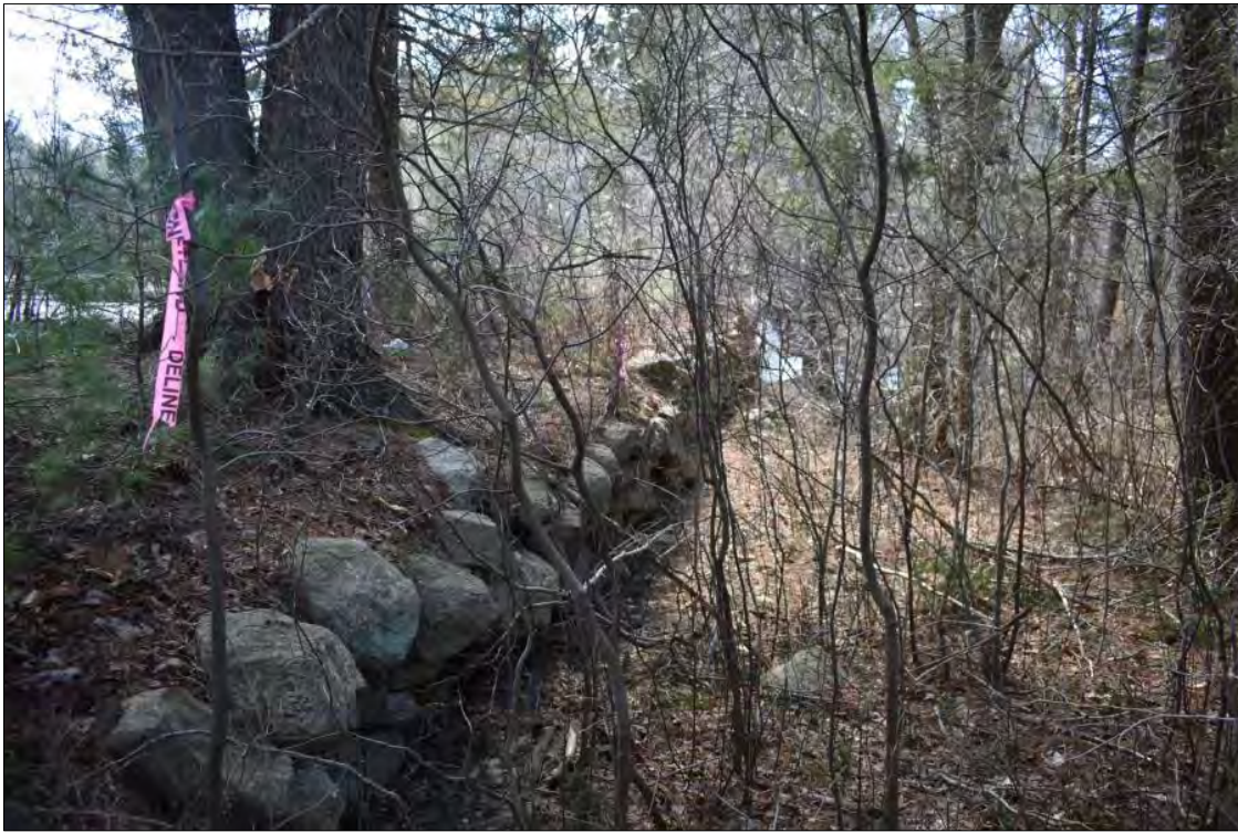
Photo 5. Dry-laid stone masonry on the downstream face of the Capwell Mill Pond Dam, view south.
